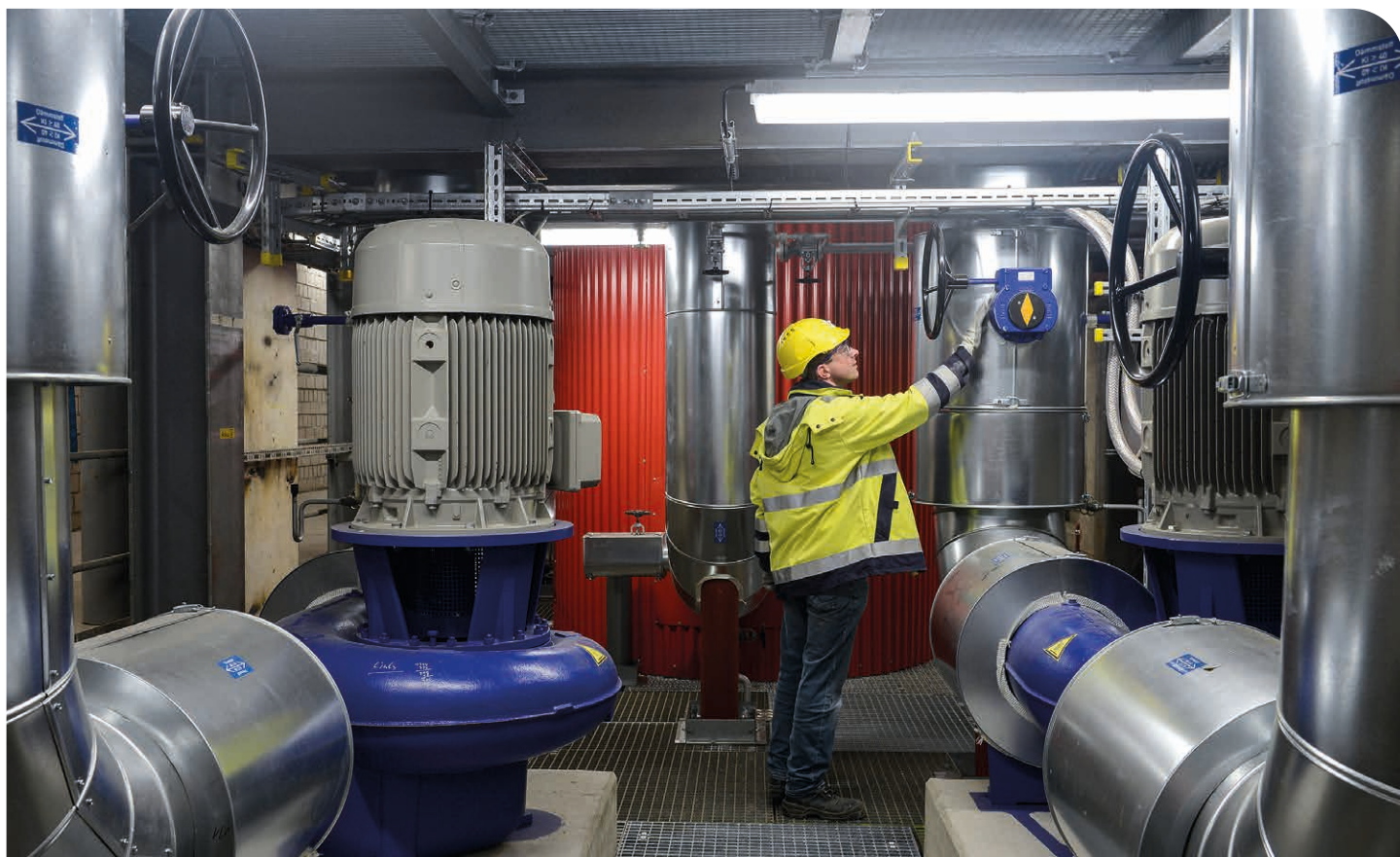
> Heat storage plant Karoline
